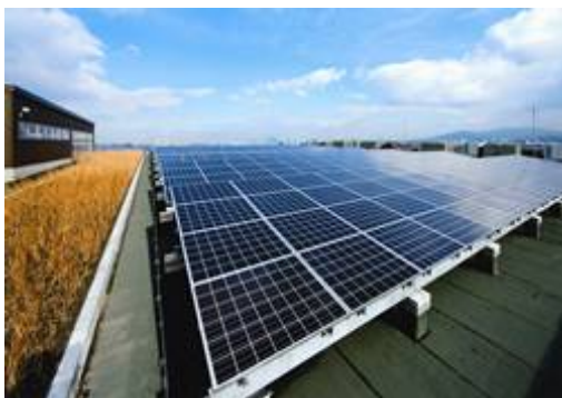
Rooftop Solar Panel 190 kW
