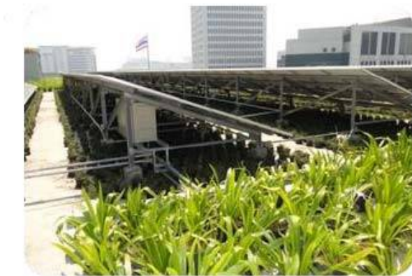
Solar Cell Panels beside Green Roof
